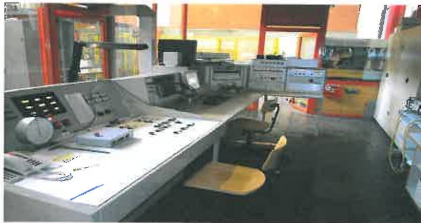
Control room for tests up to 10kA
