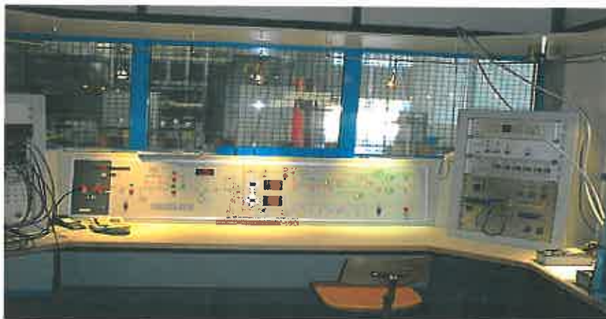
Control room for tests above 10kA
